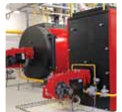
Plant Rooms and Maintenance
