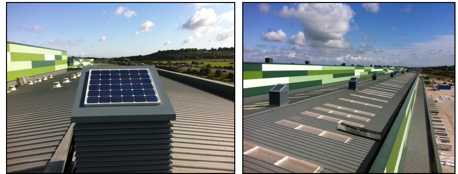
Solar Powered Roof Turrets at Morrisons Bridgwater RDC
